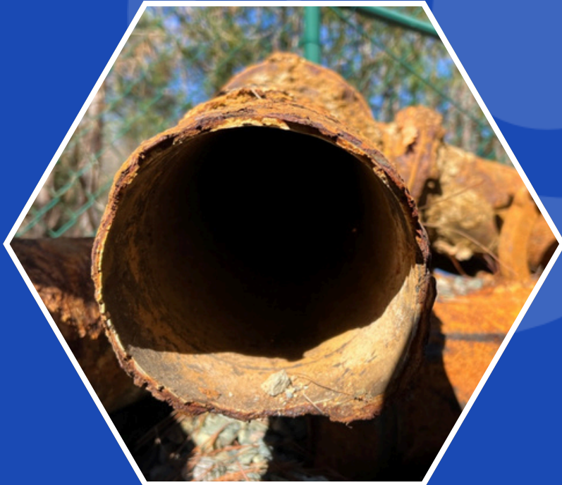
Pictured above: Piping removed from a pump station after being refurbished after only 7 years of operation. The increased rate of degradation is due to untreated sulfide in the wastewater stream.
